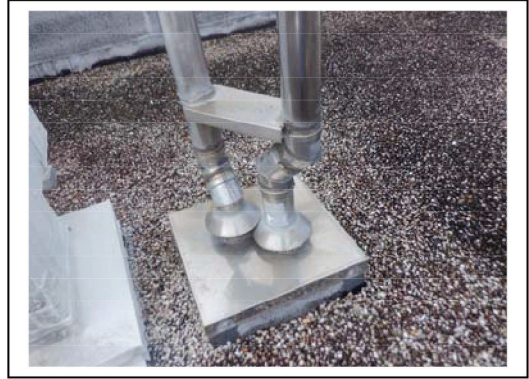
Hot Stacks on Curb
