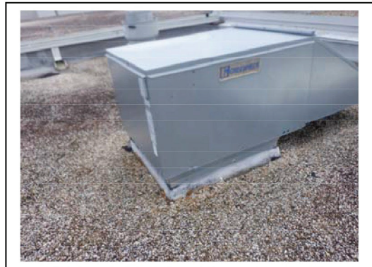
Air Intake on Low Curb
