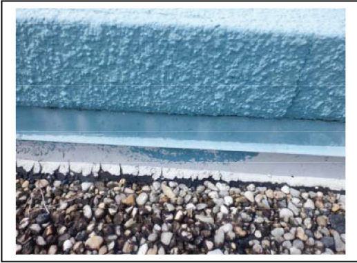
Low Base Flashing on Parapet
