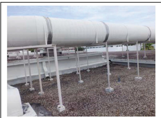
Duct on Stands
