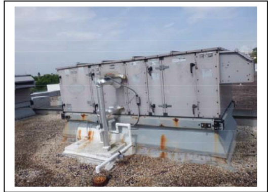
Air Handler on Curb
